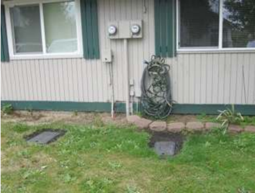
typical power meter, sewer pump alarm & water meter location @ front of buildings
