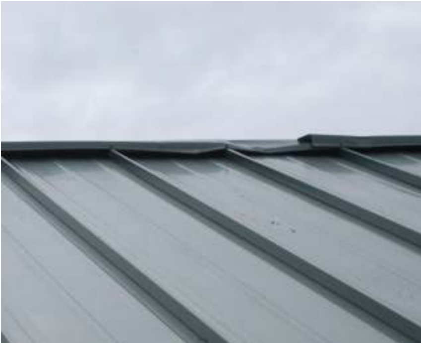
Unit 7/8 roof damage @ ridge
