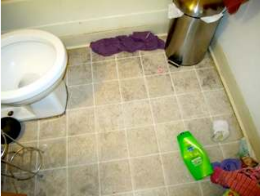
Unit 15 w/ moisture damage to bathroom flooring
