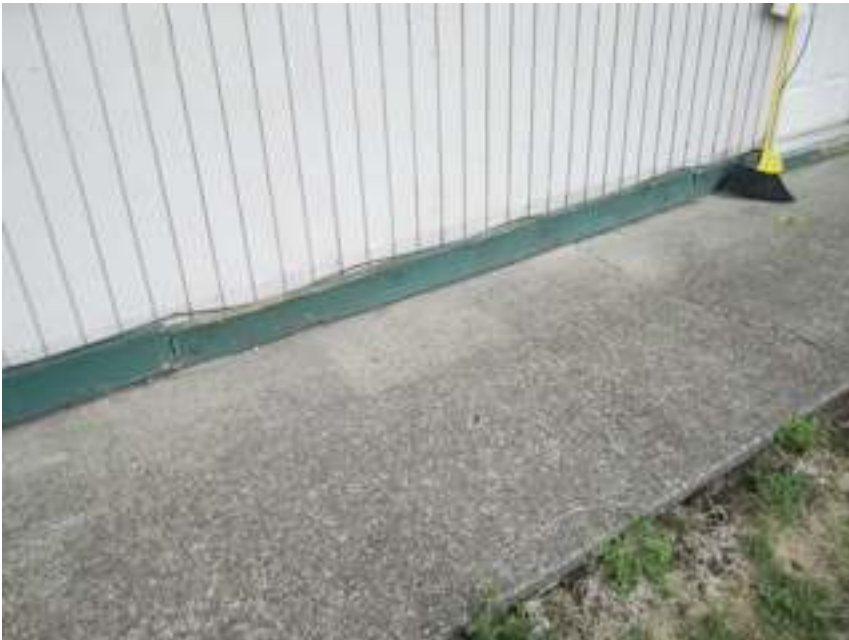
typical bellyband damage w/ decay behind trim
