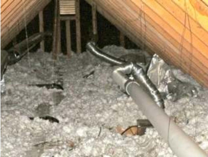
typical bath fan ducting, not to code & poorly routed
