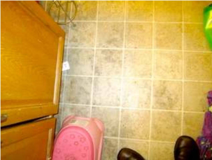
Unit 15 w/ moisture damage to bathroom flooring
