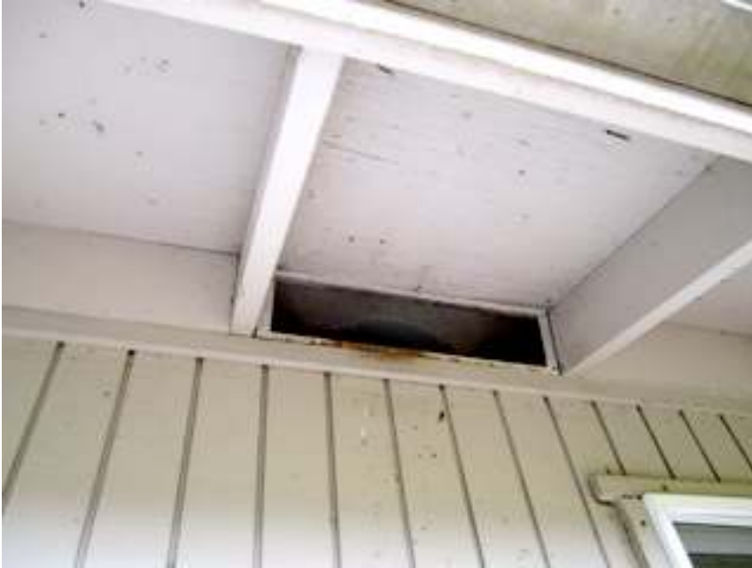
abandoned bath fan vent opening @ soffit
