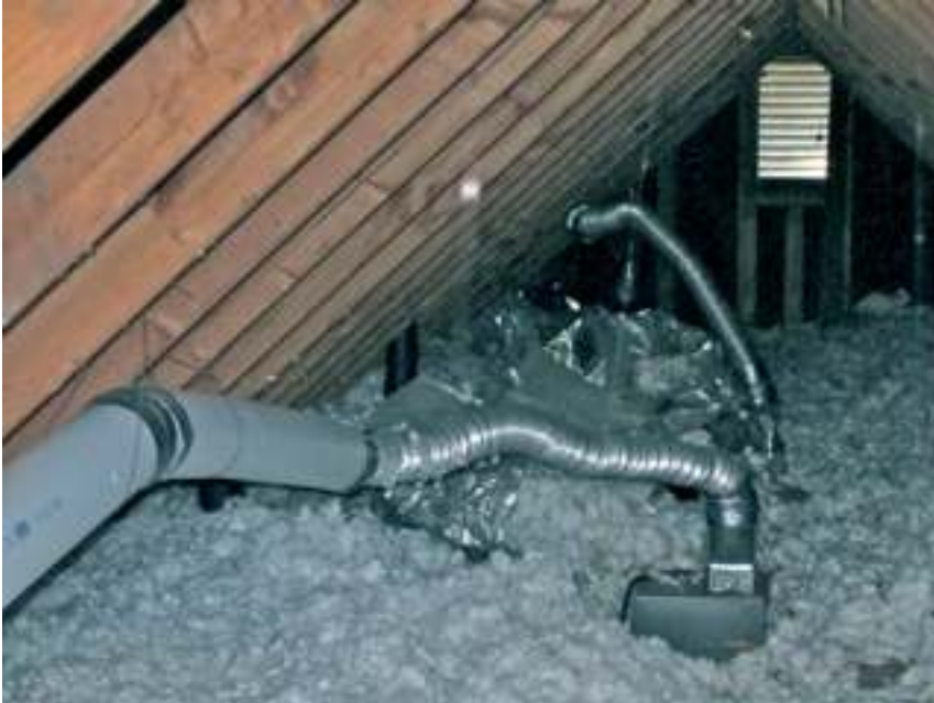
typical poor fan to ducting transition w/ missing insulation
