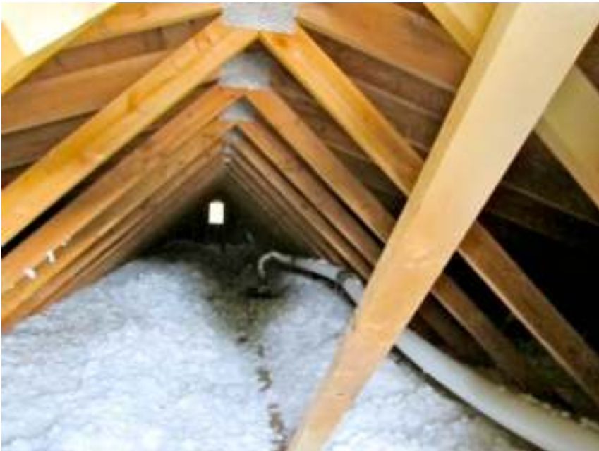
typical attic bath fan ducting poorly secured w/ low spots holding water
