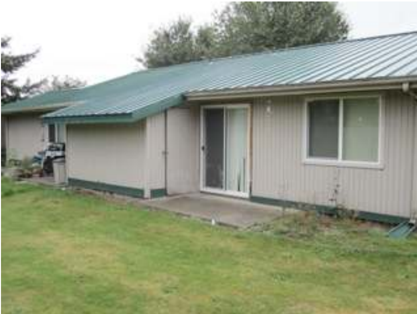
typical back side of units note extended roof line, over storage, without gutter
