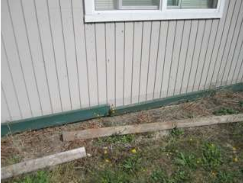
typical loose bellyband w/ fungal rot / decay behind missing flashing to prevent water behind trim
