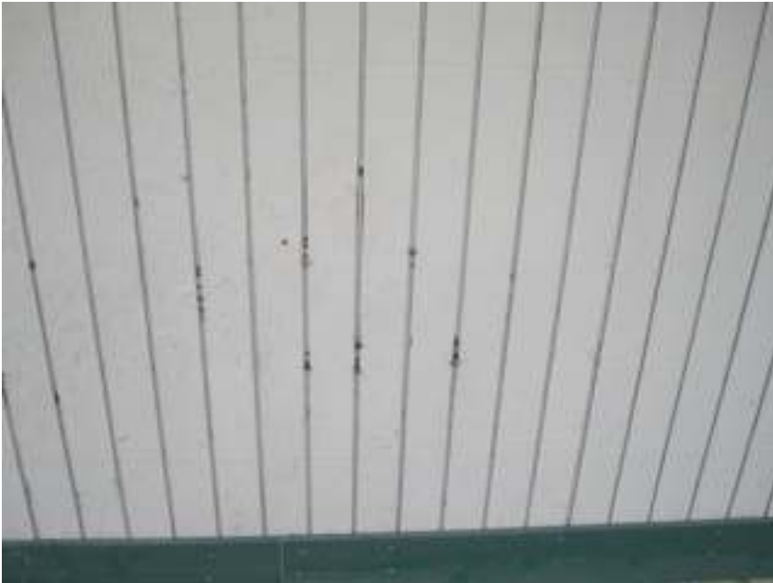
Unit 30 south wall fungi growth
