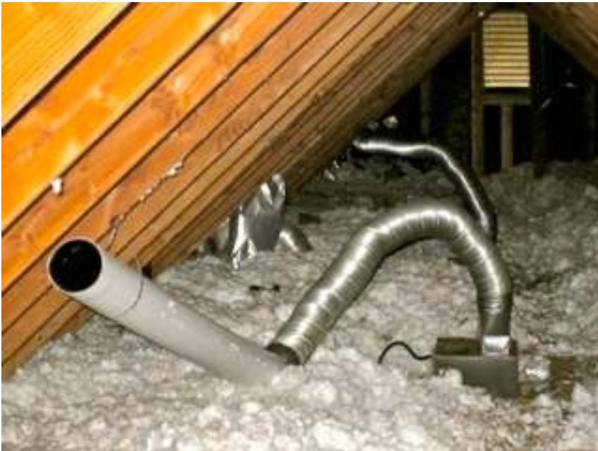
typical disconnected bath fan ducting w/ improper materials
