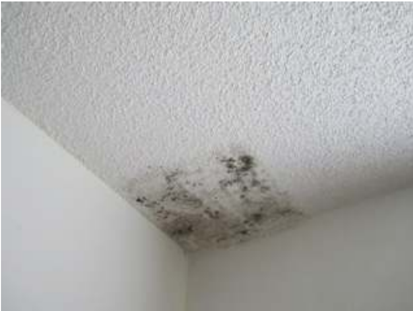
typical ceiling staining @ previous bath fan exterior soffit vent opening
