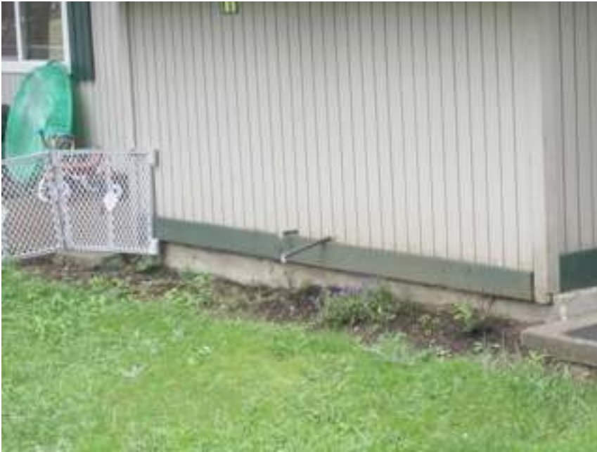
Unit 33/34 water heater PTRV's extended
