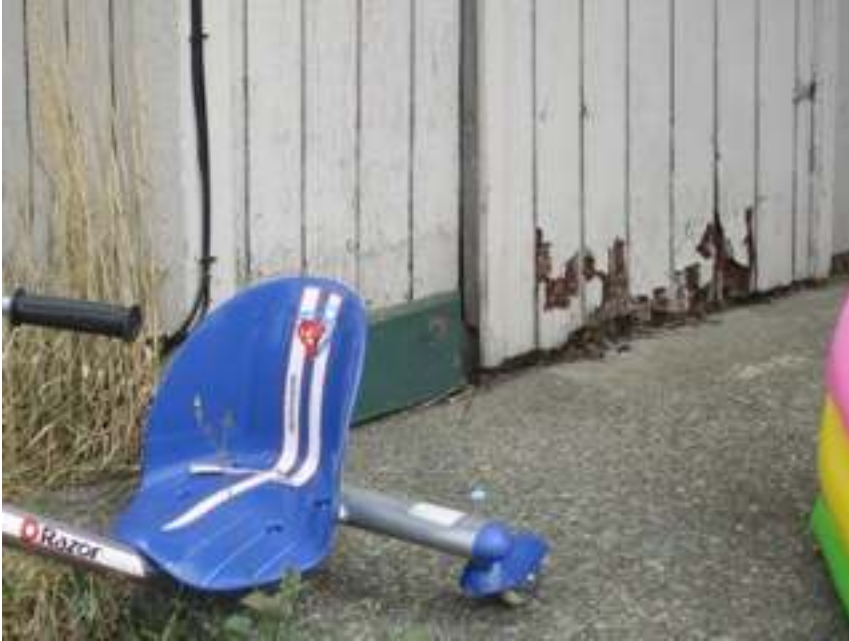
storage room door damage, typical at south facing, west side units
