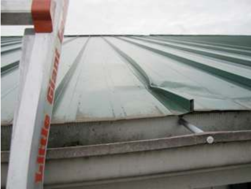
Unit 7/8 roof damage
