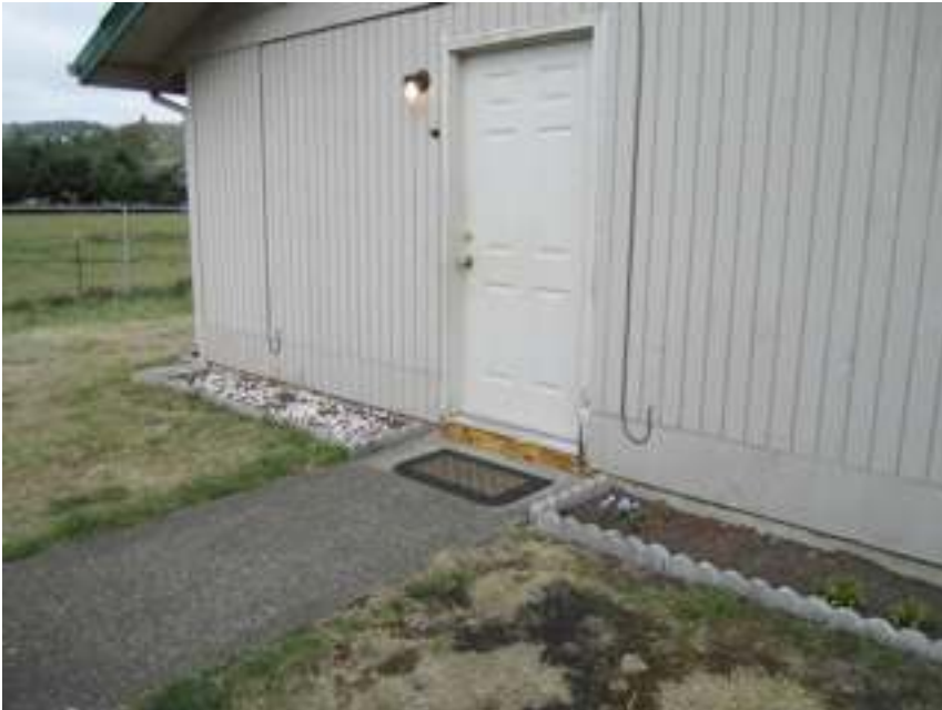
typical apartment entry, note missing threshold trim
