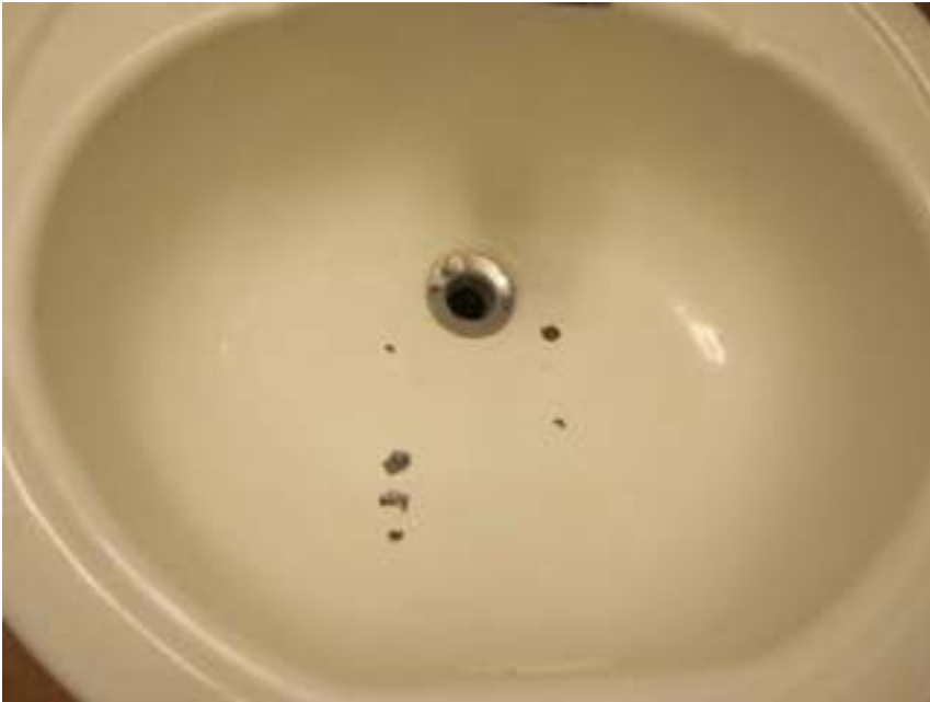
typical steel bath sink failure
