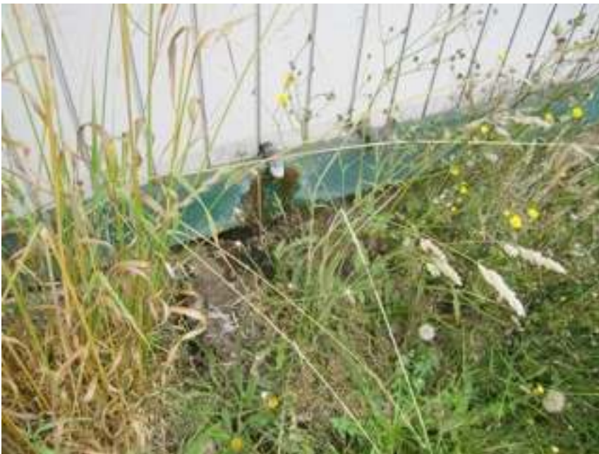
Unit 8 water heater PTRV leak
