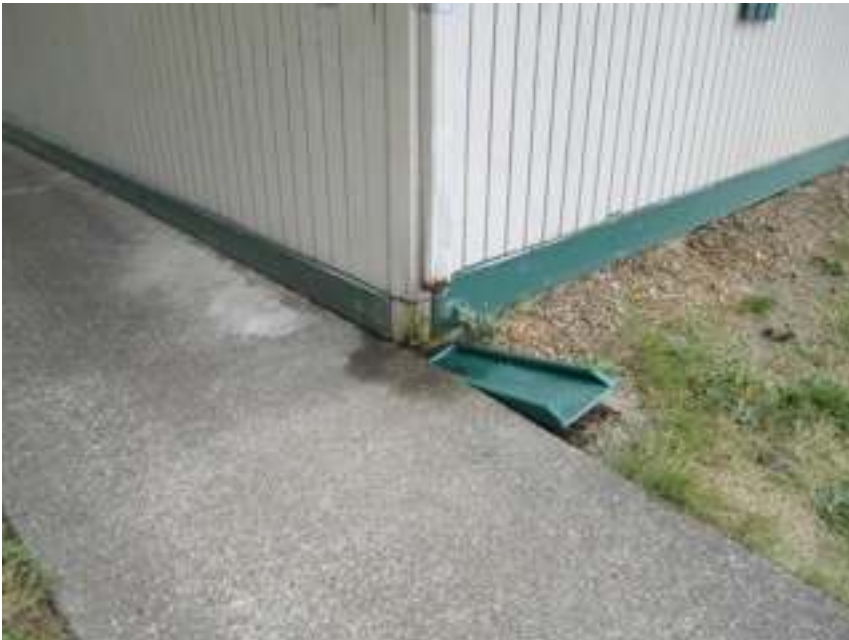
typical downspout w/ missing parts, poor splash block positioning & siding damage
