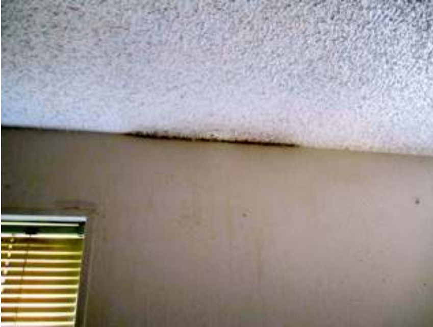
Unit 15 w/ evidence of previous very high interior moisture levels note water staining / drips on walls were observed throughout unit
