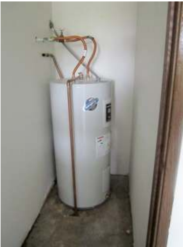
typical water heater installation, not to code
