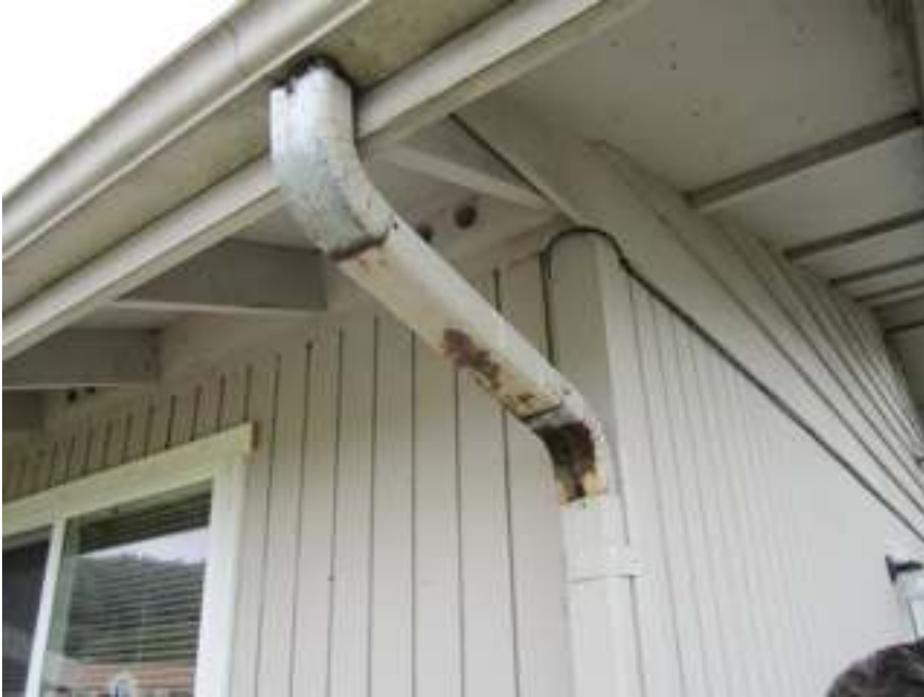
typical downspout rust
