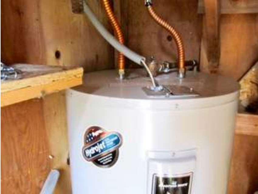
Unit 32 water heater w/ exposed wires
