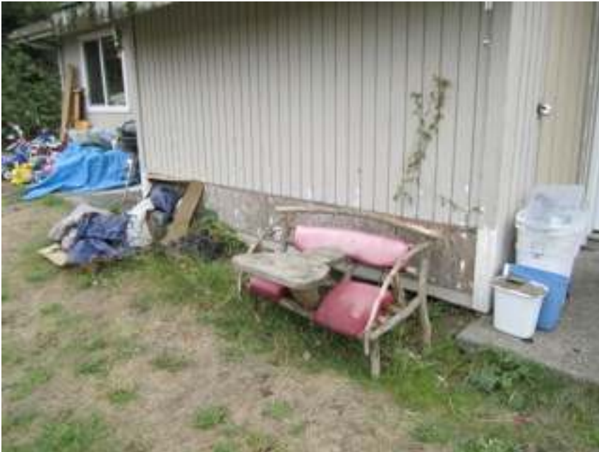
previous siding repairs to storage shed siding missing paint to prevent on going water damage
