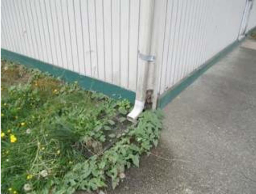
typical earth wood contact & siding damage w/ rot behind downspout
