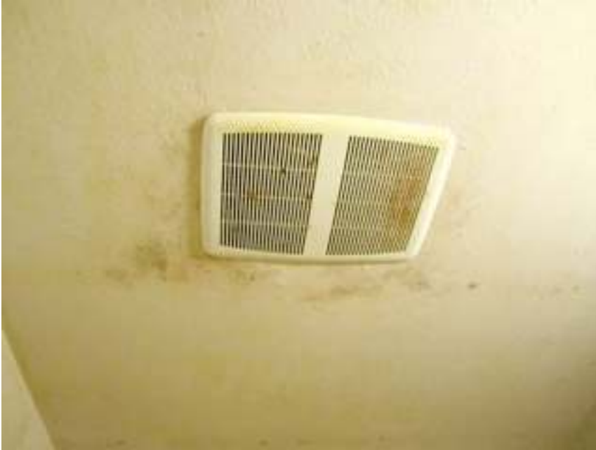
typical bath fan ceiling damage from condensate leaking due to improper ducting
