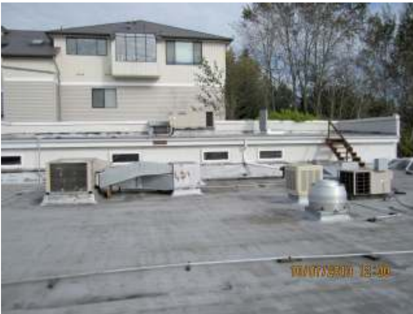
roof mounted HVAC equipment
