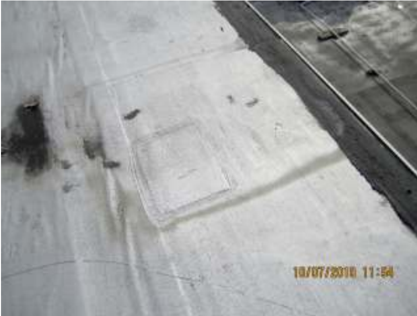
torch down roof patching & cracking
