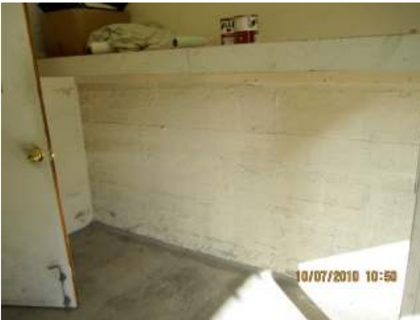
north wall water staining
