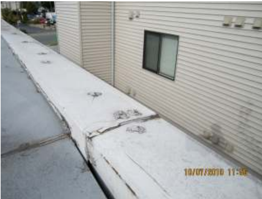
parapet wall cap flashing w/ poor / failing seals
