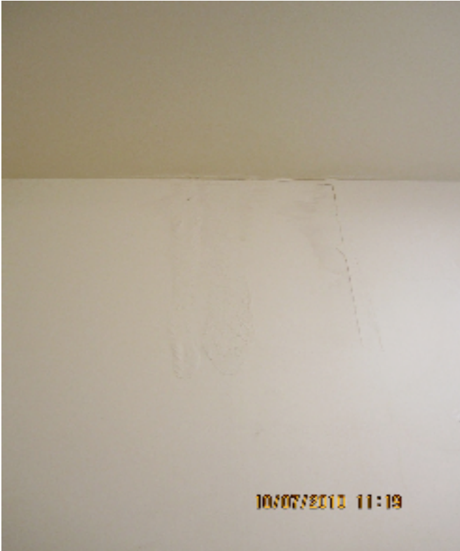
water damage below addition roof to wall intersection
