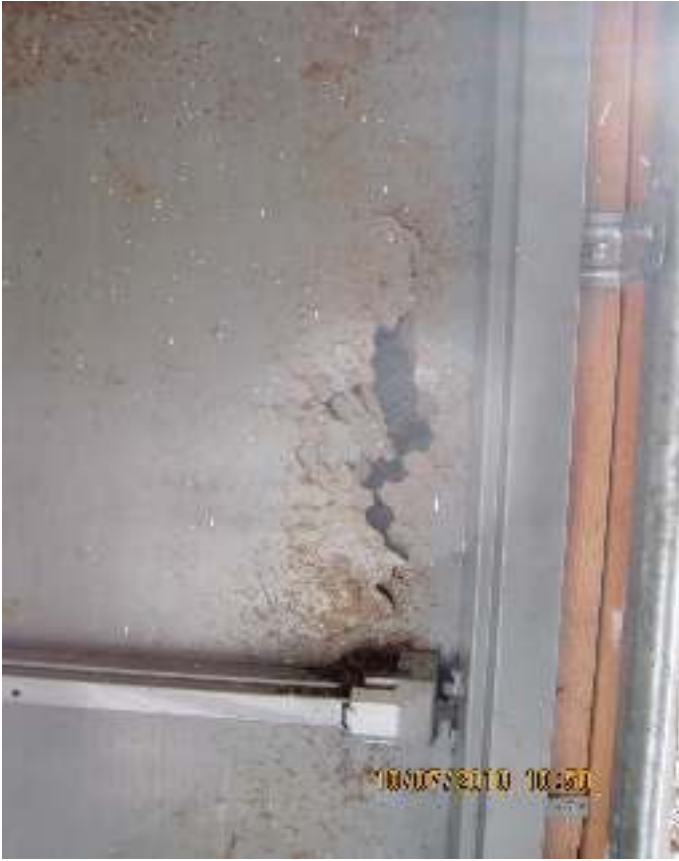
failed / rusted NE corner garage door
