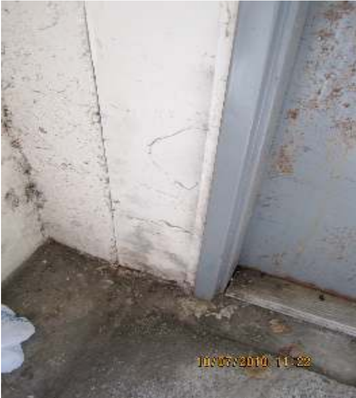
NE corner water damage & mold
