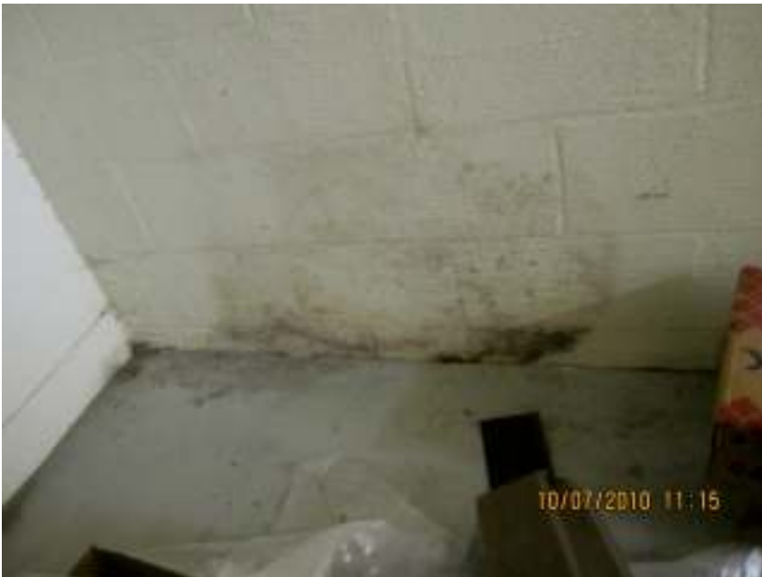
NW corner water & mold damage
