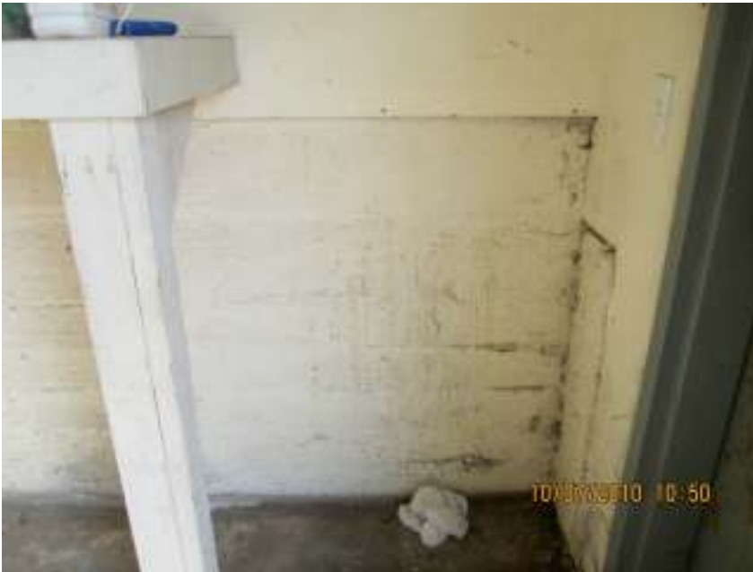
water intrusion @ NE corner
