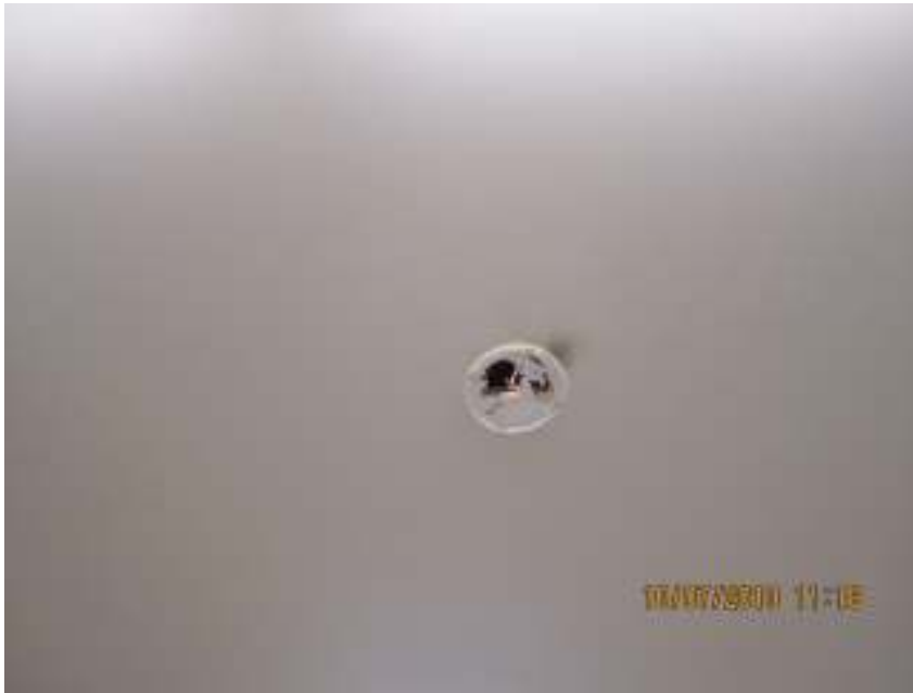
missing smoke detector
