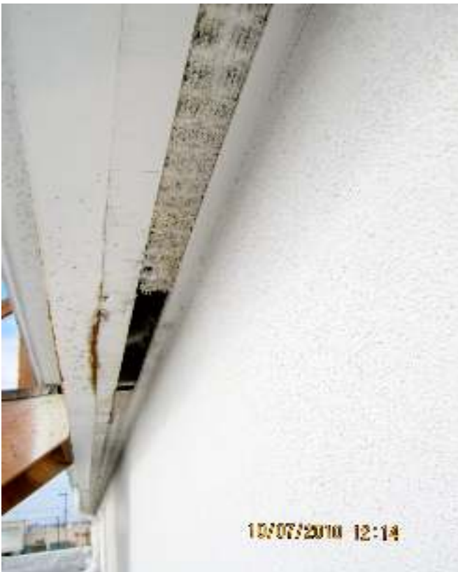
upper roof soffit corrosion, possible fan exhaust
