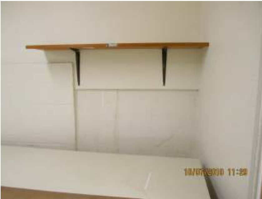
typical north wall water staining & foundation transition
