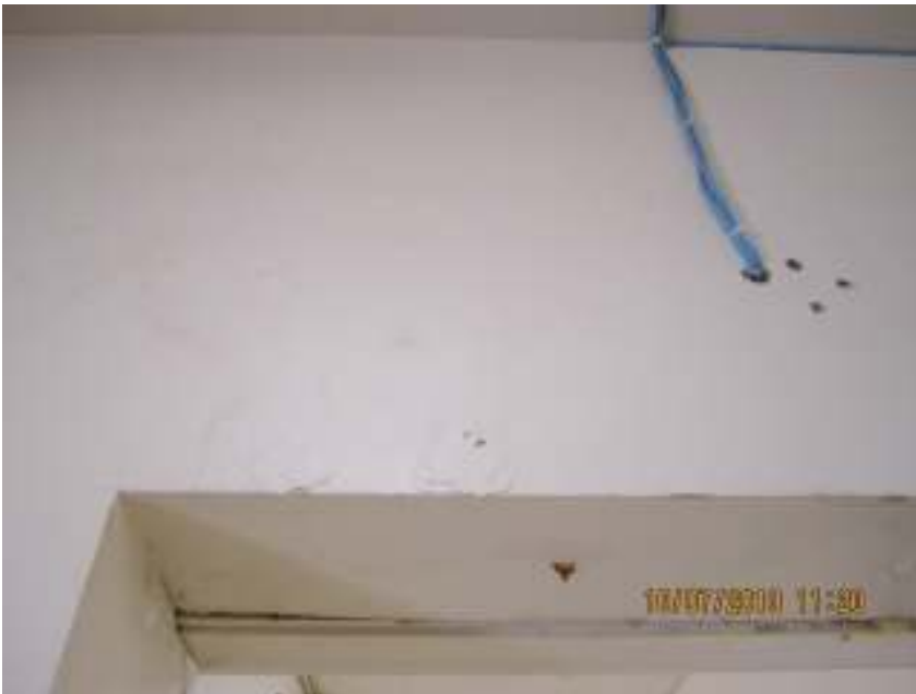
water damage below roof drain
