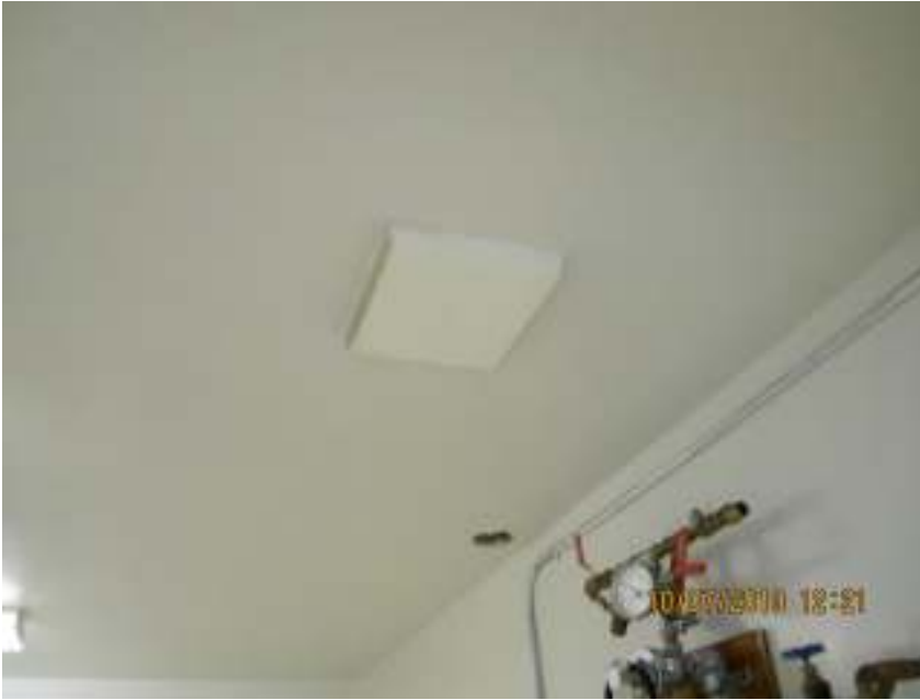
upper wet room exhaust fan w/ improper exterior venting
