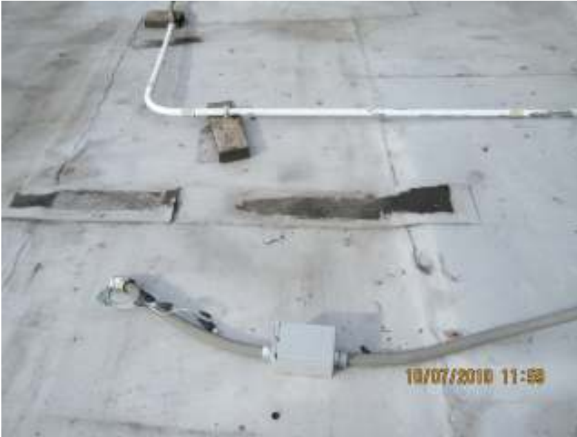
exposed electrical wiring
