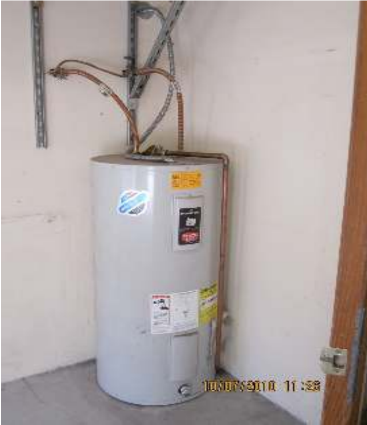
older water heater, not to code
