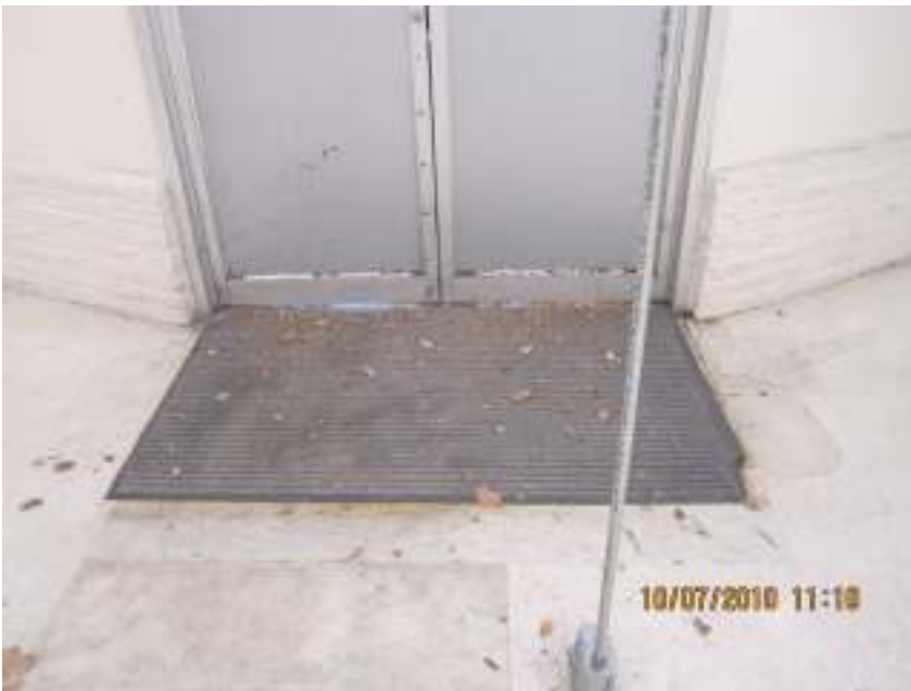
SW entry door w/ poor weather seal
