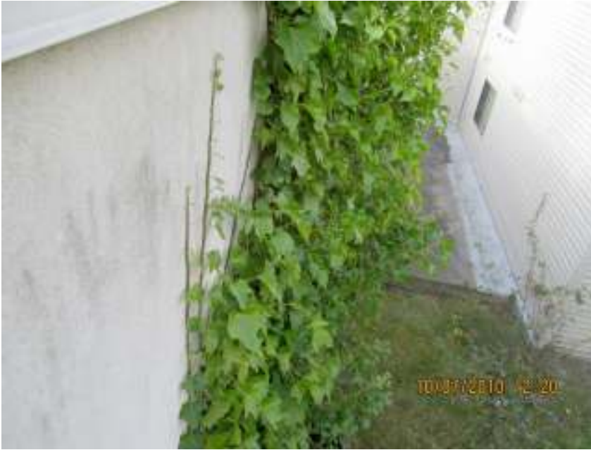
north wall ivy growth
