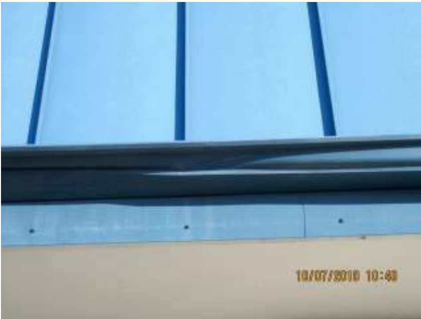
damaged gutters on south side
