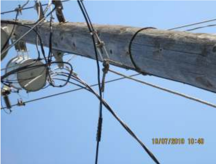
telephone wiring w/ temporary rope mounting
