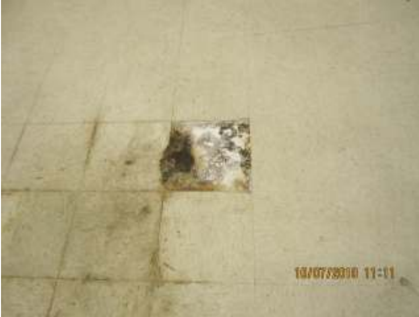
floor damage from efflorescence / moisture
