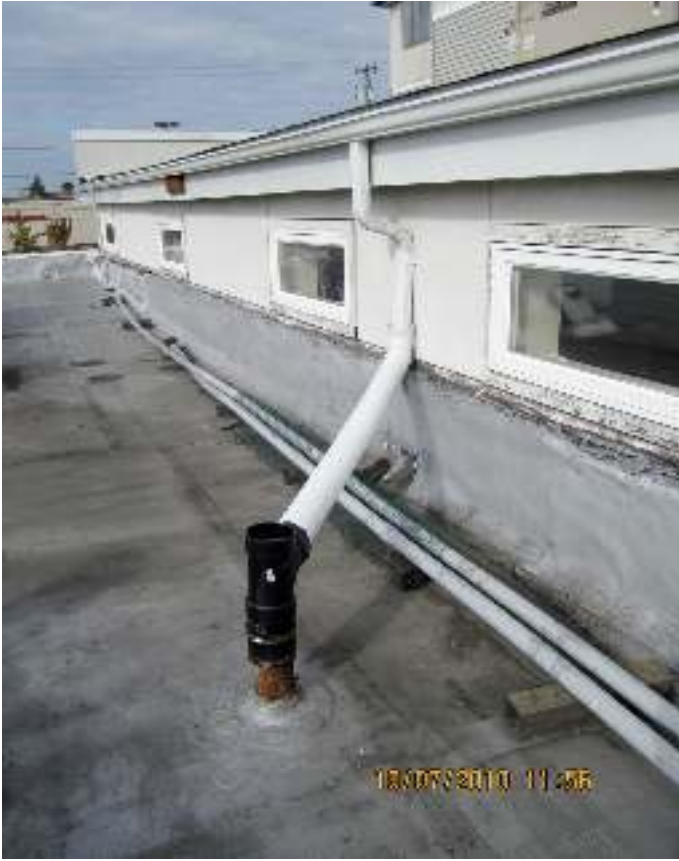
improper upper roof drain connection
