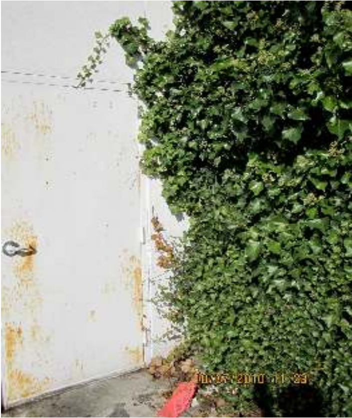
NE corner soil & ivy contact @ damage
