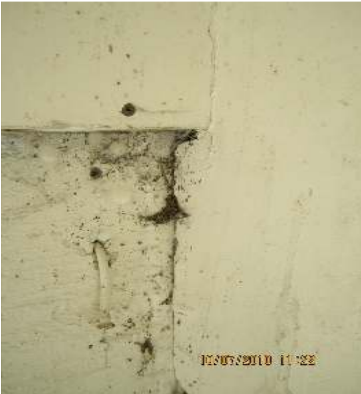
NE corner damage & ant trace
