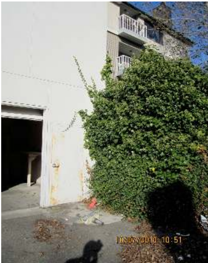
soil & ivy contact w/ exterior cladding damage
